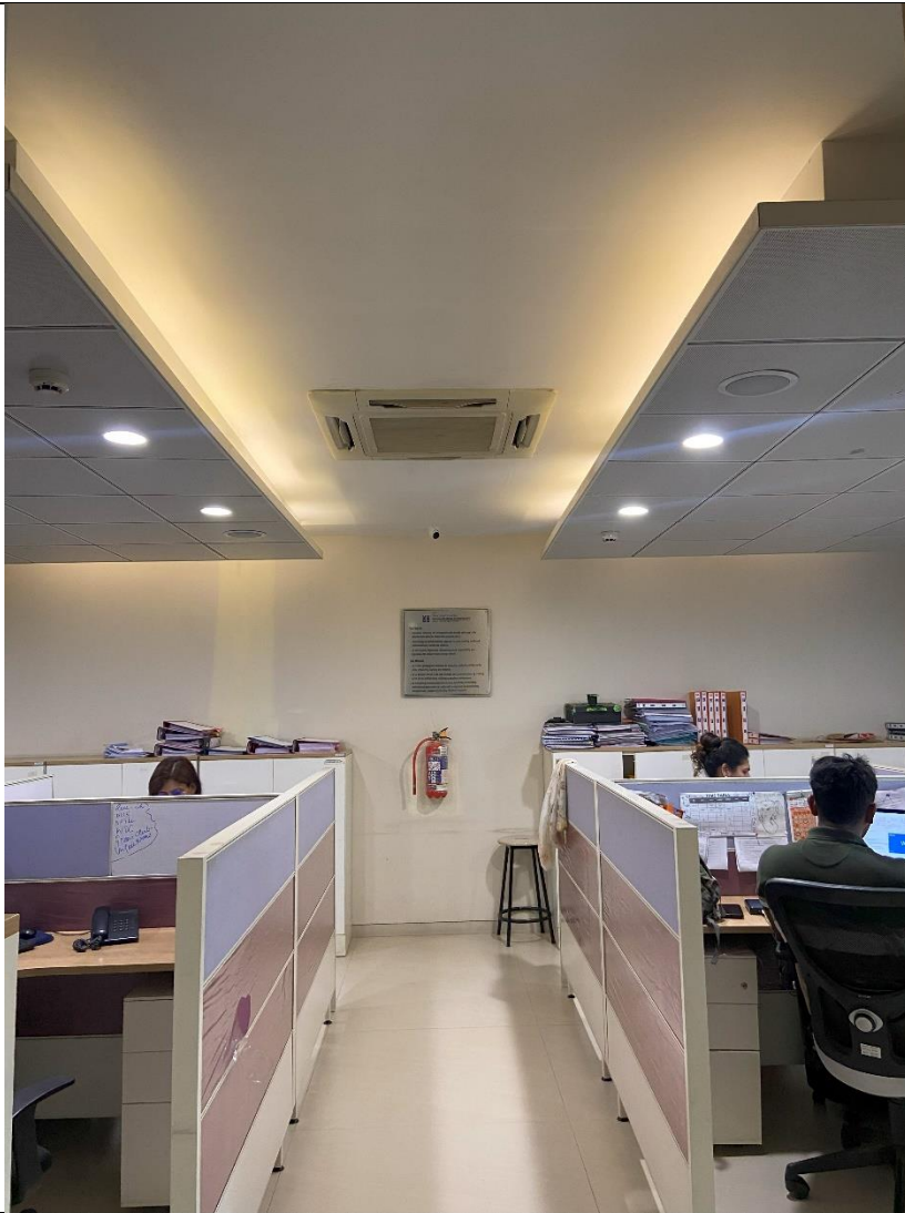
LED Panels and Lights all over the campus
